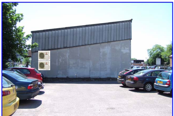
FIGURE 2 - Suggested (21.05.09) and subsequently agreed location for revised quote of £6,000 (incl of VAT fitting and grille).
