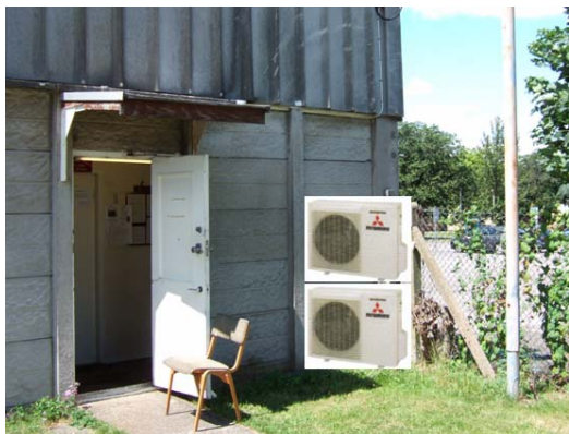
FIGURE 1b - One or two external units. Two units were confirmed (30.04.09) solution and initial proposed location.
