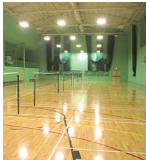
Figure 8 Note lights set in Badminton state (three luminaires only and lowered to 5 metres)
