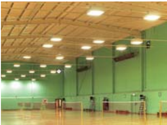
Figure 5 Note high-level radiant heaters on walls and extract fans at ends of building
