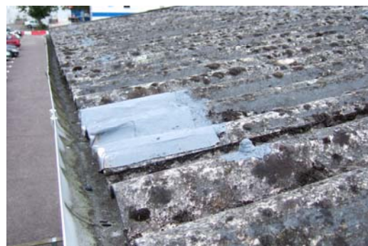
New flashing coated with sealer. Can also see sheet capping also coated. All cappings have been sealed similarly (see enlarged below).
