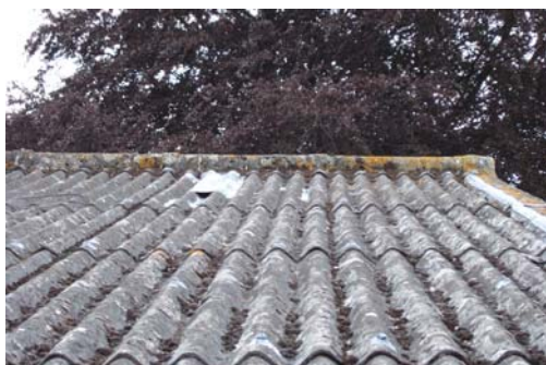
Flashing (centre) also appears to be coated with sealer. Side flashing also covered in sealer.
